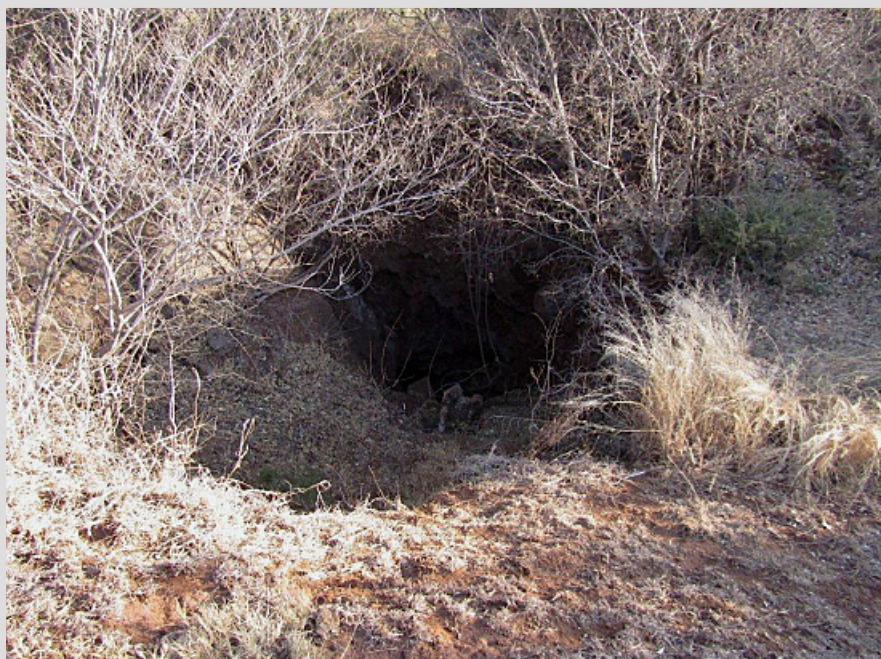
The Sinkhole at the Rock Wall
